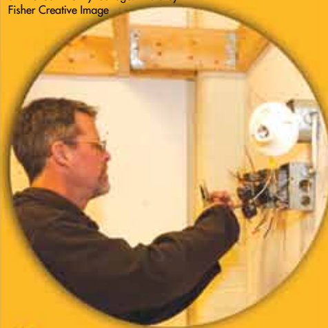
Ken Fox works on electrical wiring at Erie Community College. Photo by Fisher Creative Image
